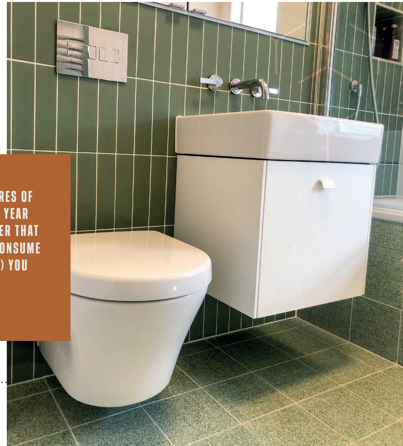
PHOTO: Water saving Toto WC installed in a new bathroom Absolute Project Management
